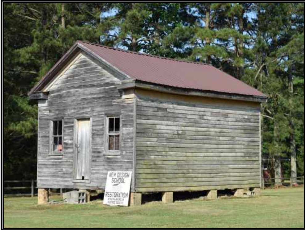
Plate 48. View of Site 090-5142, New Design School, façade and side elevation, looking northwest towards the project area.
