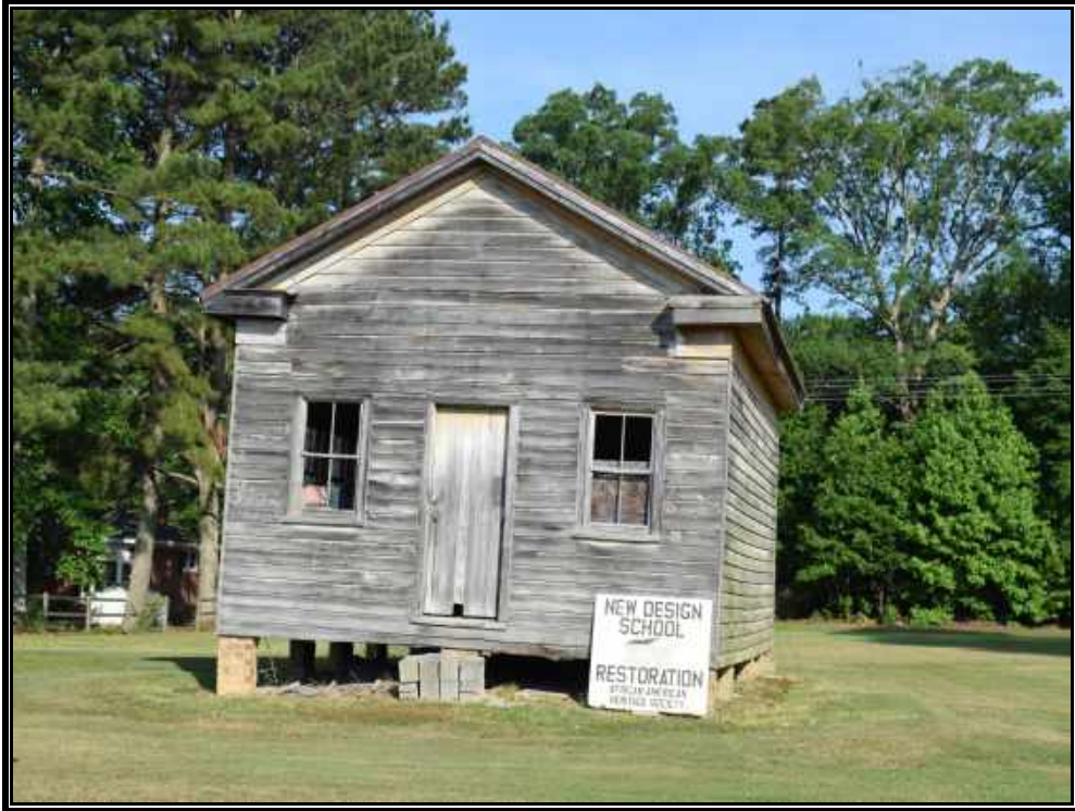
Plate 47. View of Site 090-5142, New Design School, façade and side elevation, looking northwest towards the project area.
