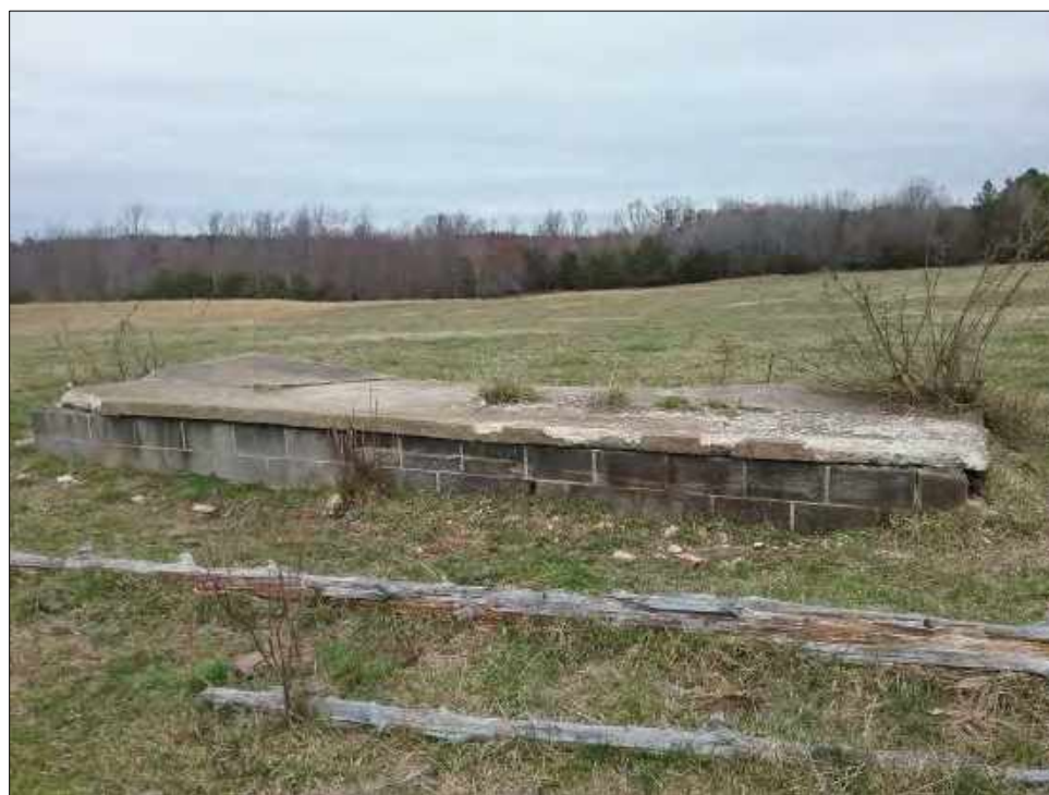
Figure 8-58: Slab associated with structural remains in area, showing cinderblocks and cement slab, facing north.
