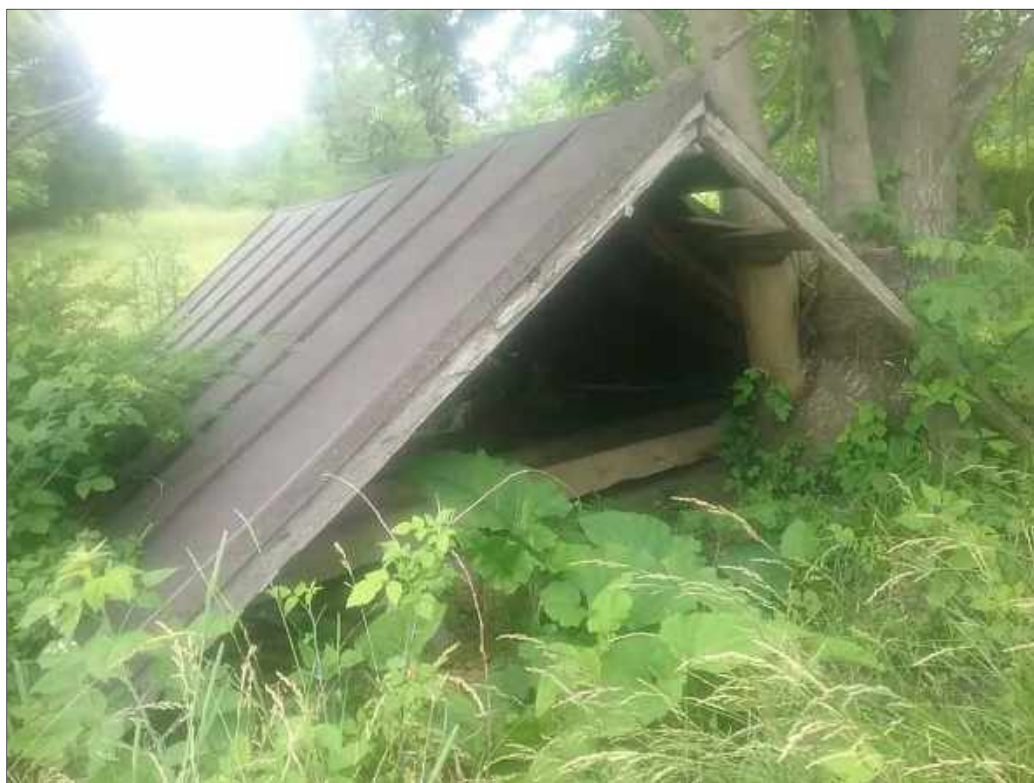
Figure 8-30: Collapsed shed, facing southwest.
