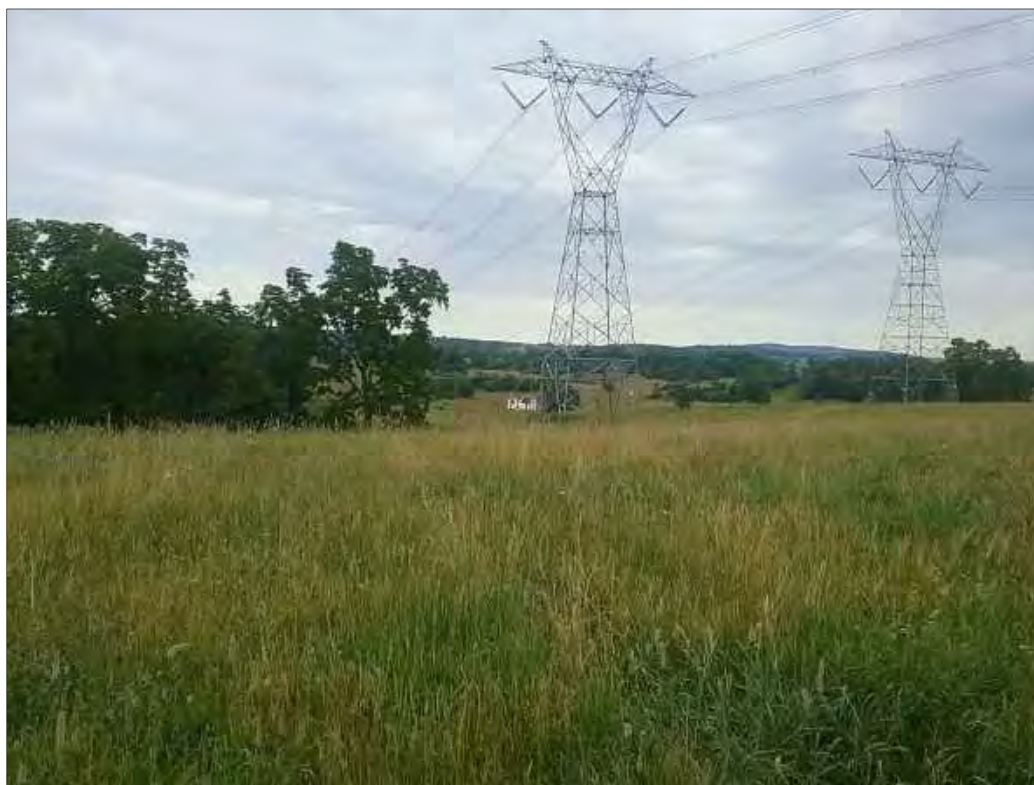
Figure 8-51: Powerline in the northern portion of Area K, facing north.
